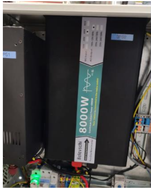
Fig. 2. Belevschi 8000W inverter
