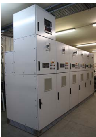
Fig. 2. The appearance of the six sections of the LV switchgear
