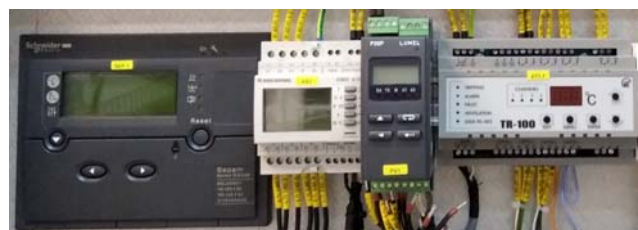
Fig. 6. View of the distribution of protection and measurement automation systems in the switchgear cell
