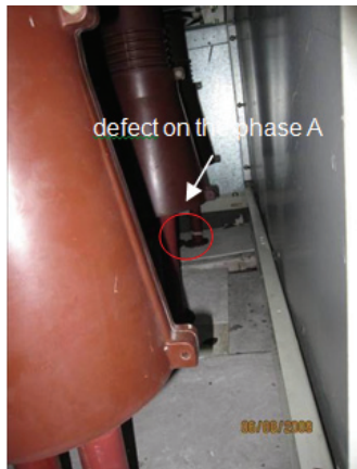
Fig.12 Photos of defective cable termination
